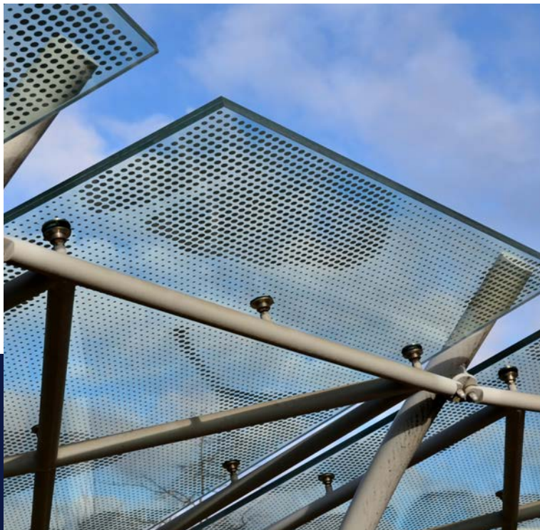
Laminated Glass Overhead Canopies
